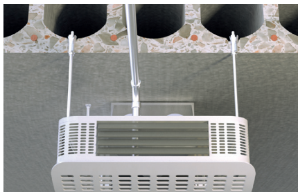
Aircondition i forspente hulldekker
