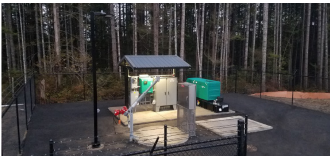
Application example: Wastewater lift station with generator set supply
